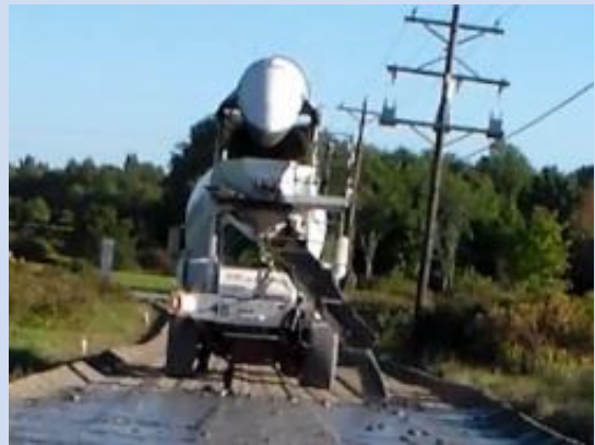
Cement Slurry is a mix of cement and water that is applied in a liquid form to the ground roadway base during full depth reclamation projects to provide base stability.
