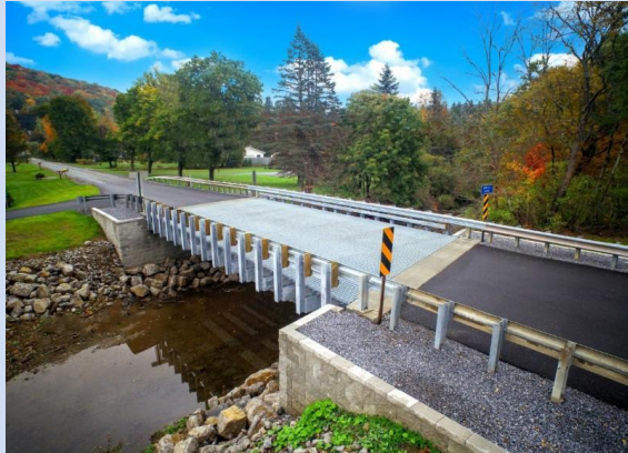
Several bridges across the state have been using the GRS-IBS technique, including a bridge project in McKean County.
