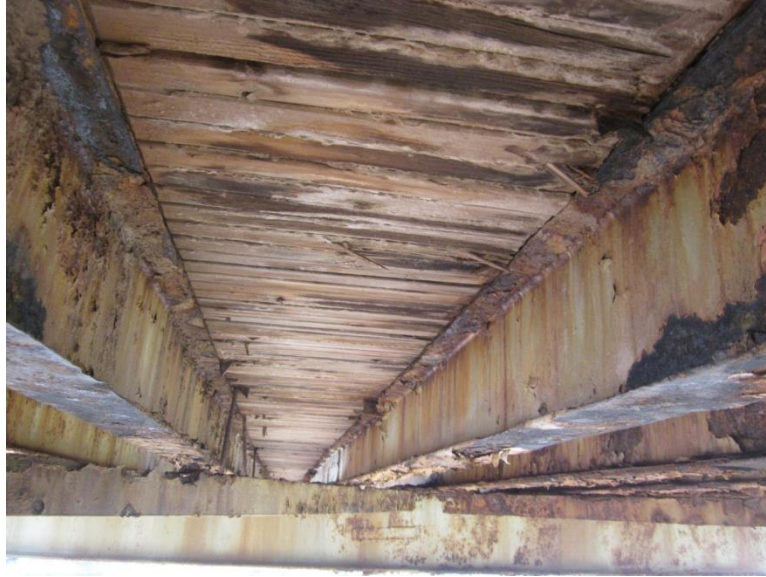
Photo 19 - Skidders Falls Bridge: Typical deck underside condition. Note missing clips
