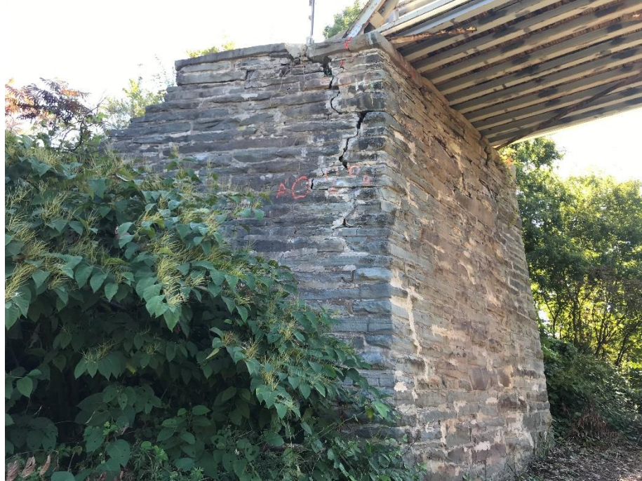
Photo 23 - Skinnners Falls Bridge: Far Left Wingwall with Crack Monitoring Points and Full Height Step Cracking
