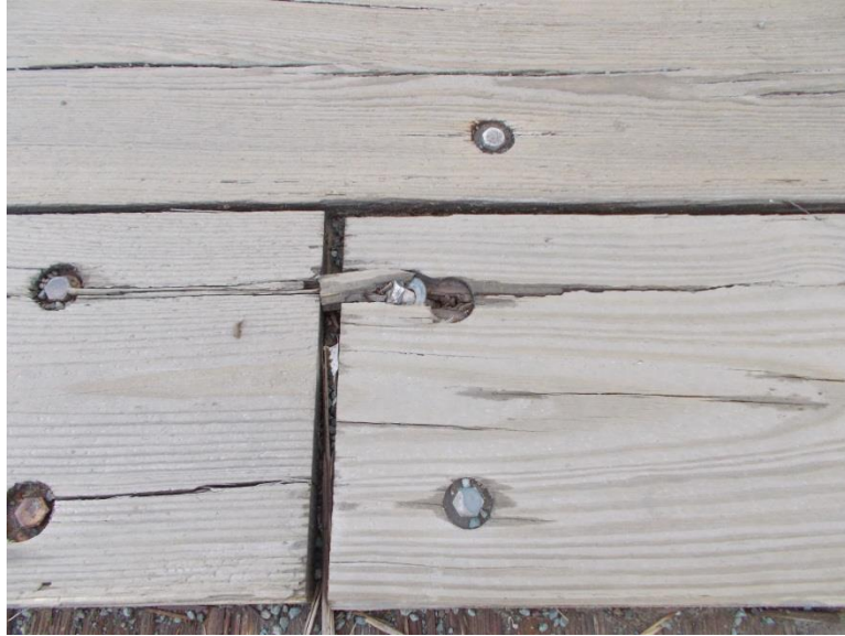
Photo 35 - Skidders Falls Bridge: Typical Damaged Tread Connection (Span 2 Shown)
