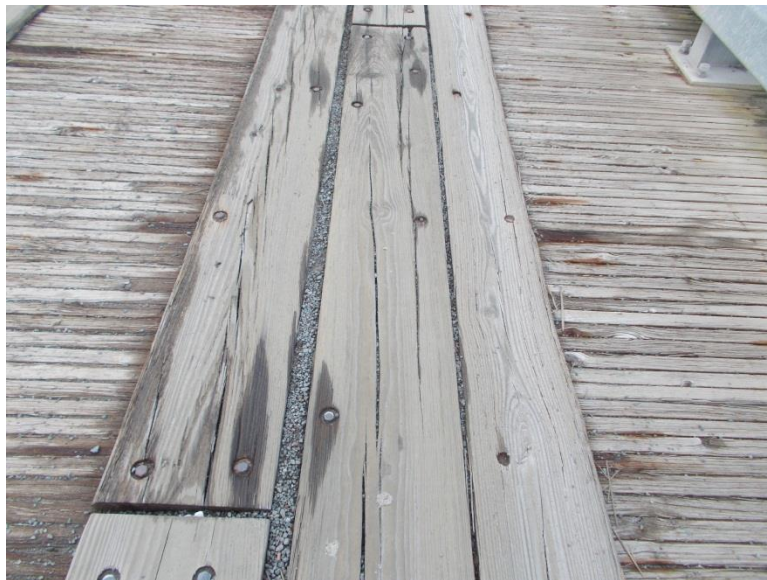
Photo 34 - Skinners Falls Bridge: Typical Cracks and Splitting Throughout Left Tread
