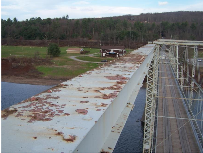
Photo 9 - Skinnners Falls Bridge: Left Truss Top Chord flaking paint and minor surface rust
