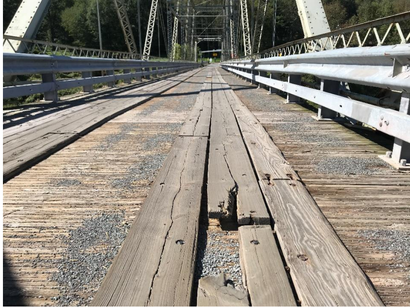
Photo 5 - Skiners Falls Bridge: Timber Running Board Deterioration
