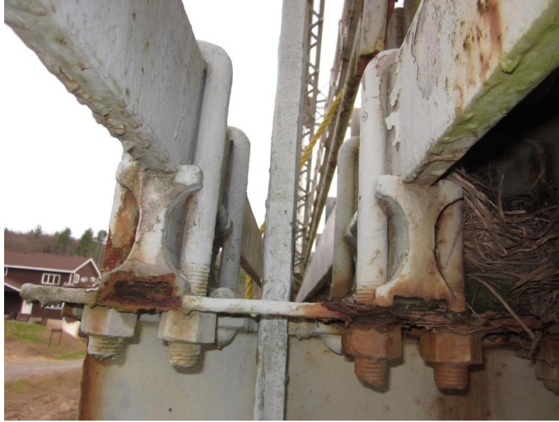
Photo 21 - Skinnners Falls Bridge: Floor Beam Support deterioration
