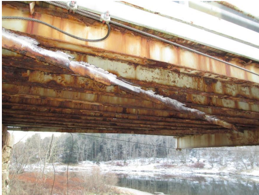
Photo 22 - Skinnners Falls Bridge: Span 2, Floor Beam Bay 12, 100% section loss to bottom lateral bracing
