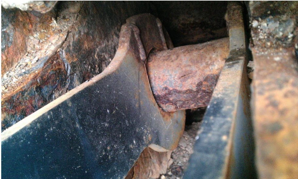
Photo 16 - Skidders Falls Bridge: Existing field welded s to lower chord forged eyebar heads
