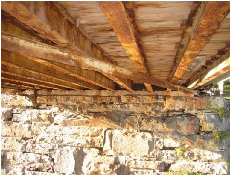
Photo 26 - Skinnners Falls Bridge: Near Abutment with wide mortar joints with deep voids at the top half
