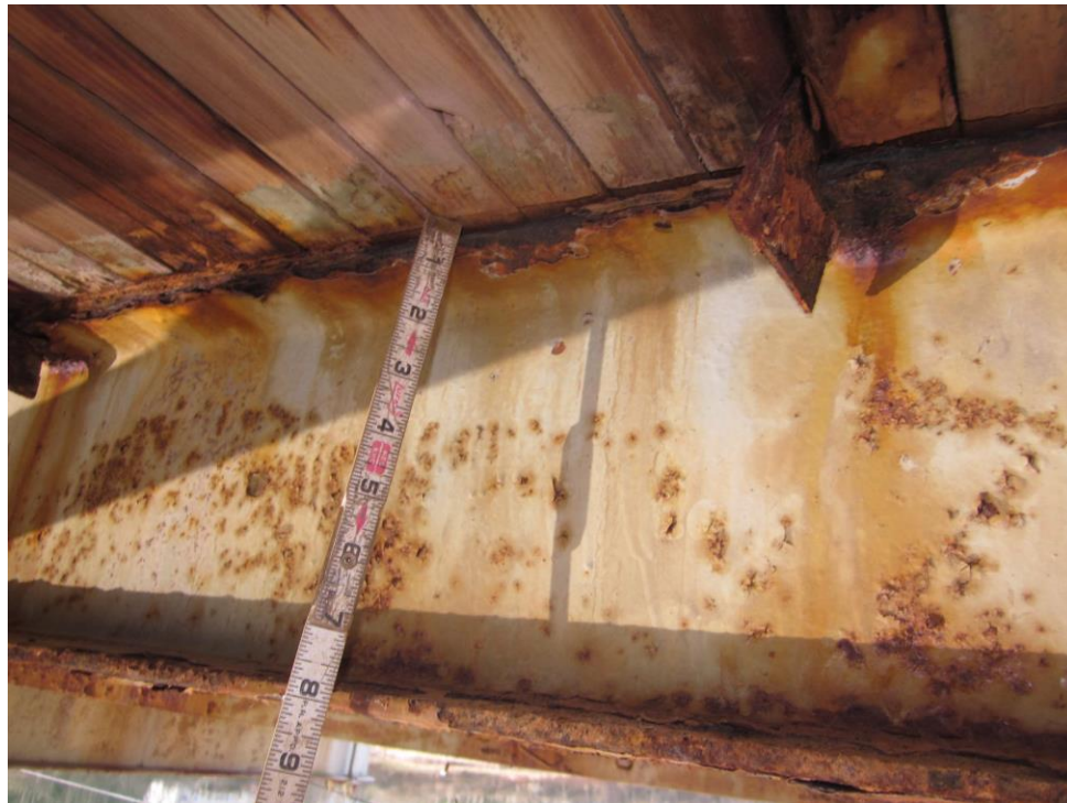
Photo 20 - Skidders Falls Bridge: Gap between stringer and deck due to section loss
