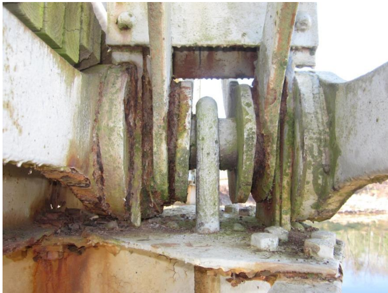
Photo 18- Skinnners Falls Bridge: Span 2, Left Truss, Panel Point L6 extensive pack rust (Looking Back)
