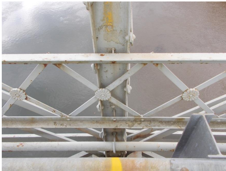
Photo 38 - Skidders Falls Bridge: Railing Bolted to Vertical Truss Member, Span 2
