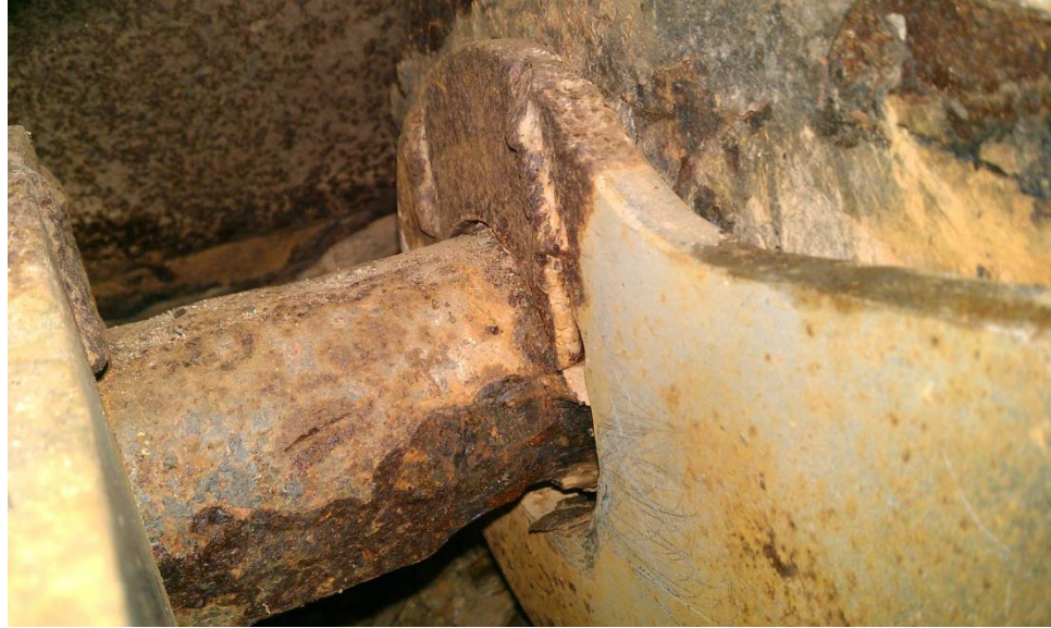
Photo 15 - Skidders Falls Bridge: 1/4" Section Loss to one side of pin at Span 1, Left Truss, Panel Point L0 (Looking Back)
