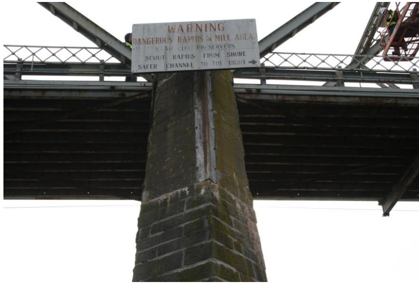
Photo 27 - Skinnners Falls Bridge: Steel Cap at the Top of the Upstream Nose of Pier
