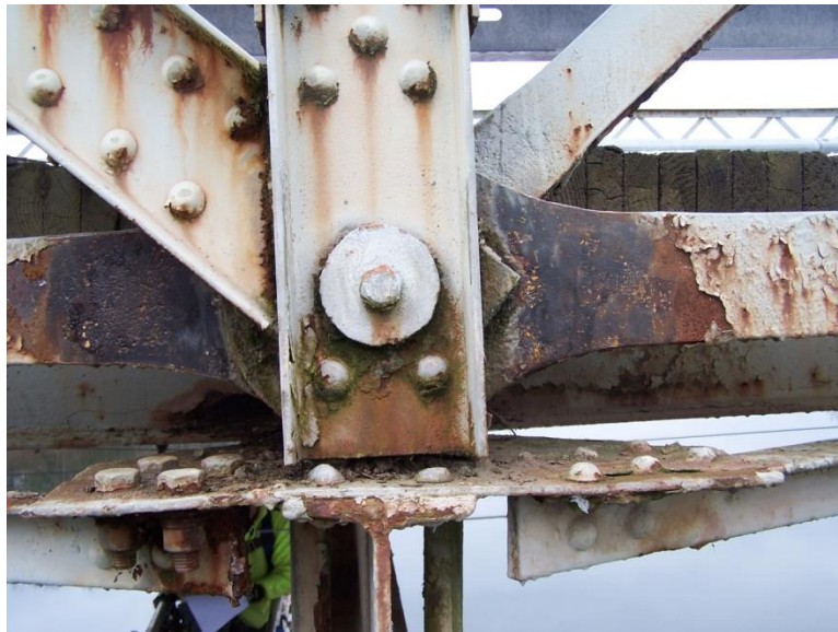
Photo 14- Skidders Falls Bridge: Span 1, Right Truss, Panel Point L8 retrofit pin cap (Looking Left)
