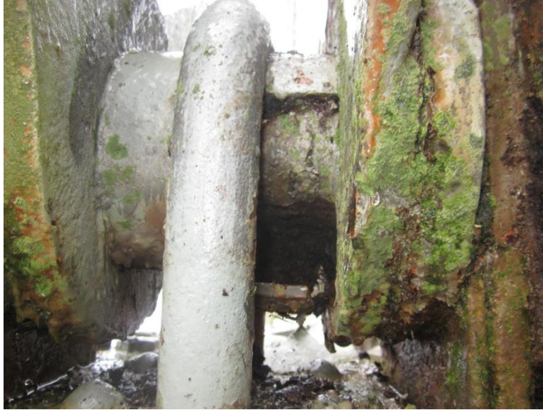
Photo 17 - Skinnners Falls Bridge: Span 1, Left Truss, Panel Point L6 pin sleeve broken (Looking Ahead)
