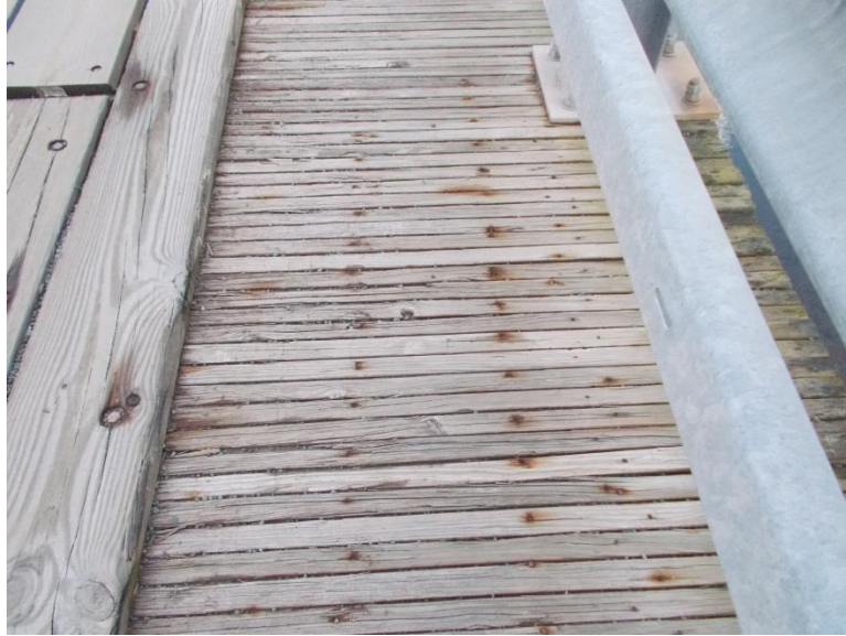
Photo 33 - Skinners Falls Bridge: Typical Deterioration of Left Edge of Deck.
