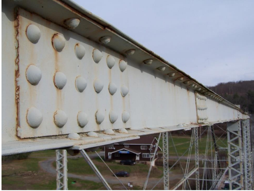
Photo 11 - Skinners Falls Bridge: Bent and misaligned bolts in top chord splices in Span 2 resulting in displacement of top chord channels.
