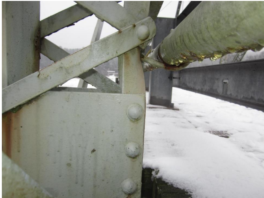
Photo 12 - Skinners Falls Bridge: Collision damage to vertical members at deck level behind the bridge railing
