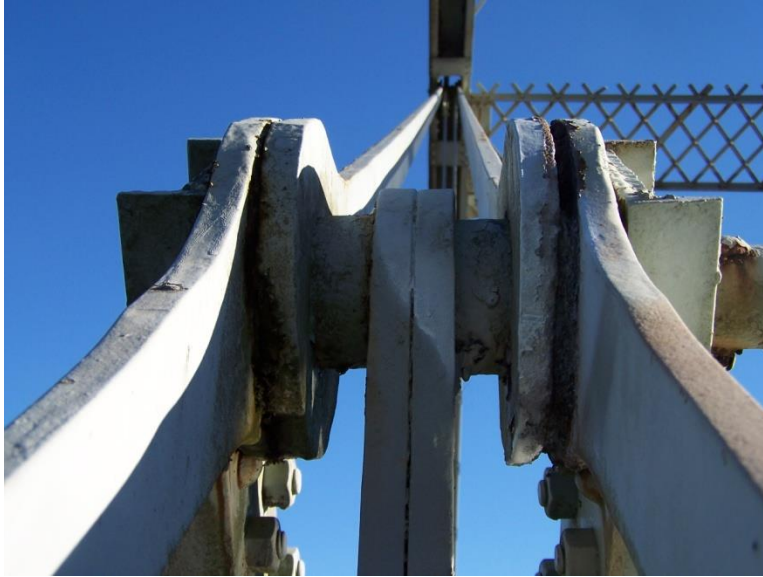
Photo 13 - Skidders Falls Bridge: Typical losses to eyebar heads at middle panel points
