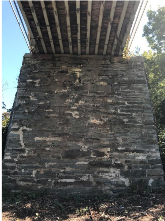
Photo 25 - Skinnners Falls Bridge: Far Abutment with Crack Monitoring Points and Full Height Step Cracking
