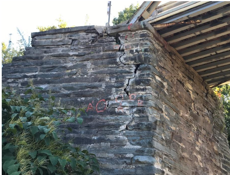
Photo 24 - Skinnners Falls Bridge: Far Left Wingwall with Crack Monitoring Points and Full Height Step Cracking
