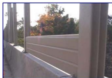
Construction of the Carsonite sound wall system on I-78 bridge over Veracruz Road
