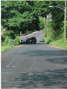
Post-construction view of the Jefferson Street Project, from the eastern boundary facing west
