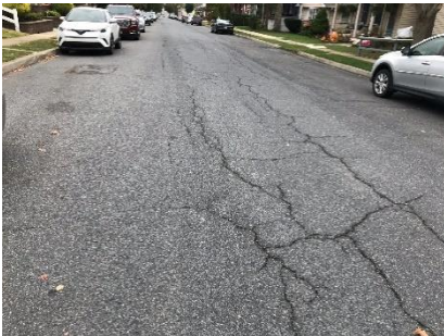
View of longitudinal cracking observed at the Hay Terrace Project
