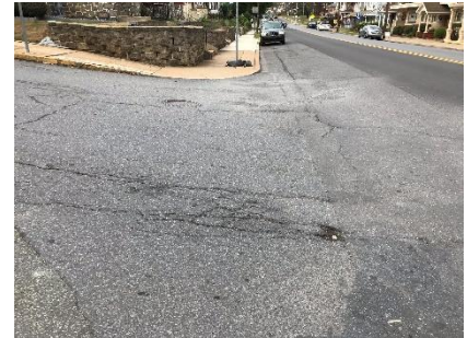
View of cracking and potholes observed along the northern boundary of the 21 st Street Project
