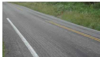
Surface bleeding observed during the one year evaluation of the Allegheny County Project Site
