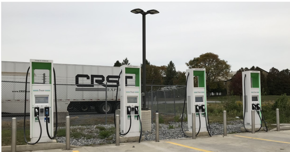
FIGURE 2: Electrify America Station at Sheetz #191 in Carlisle, PA (I-81 Exit 52)
