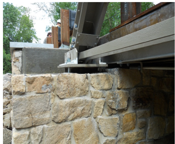
Rehabilitated Bearing with Rollers Removed and Replaced with a Neoprene Bearing Pad.
