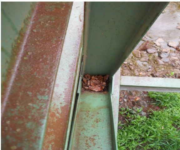
Typical Debris Accumulation at Lower Chord Joints.
