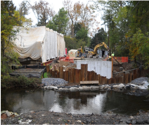
Truss Relocated to Side While New Abutments Constructed. Note Paint Containment System.
