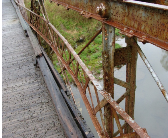
Vehicular Impact Damage to Ornamental Bridge Railing.
