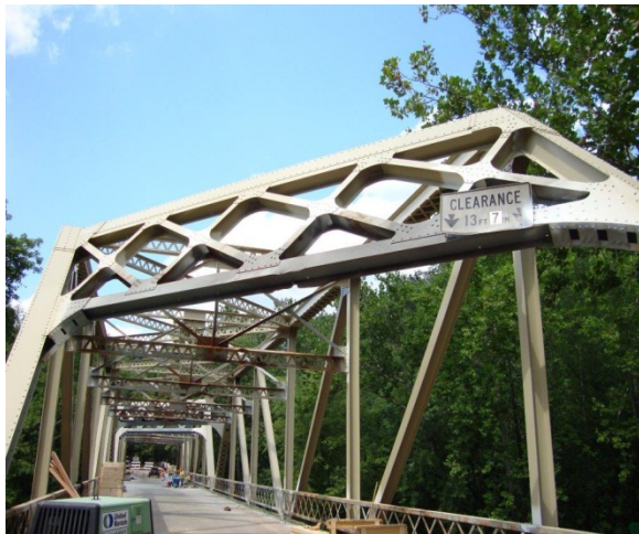
Substandard Vertical Clearance with Portals and Bracing Existing Collision Damage.
