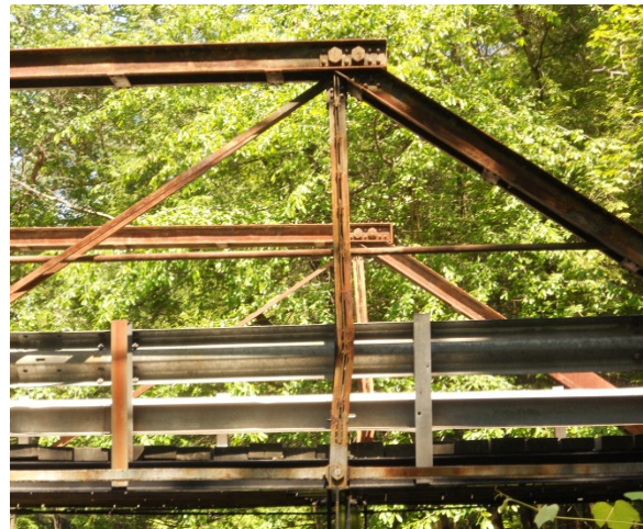
Truss Vertical with Vehicular Impact Damage Prior to Guiderail Installation.
