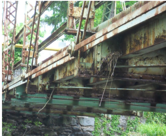
Flood Debris on Lower Chord and Floor System.
