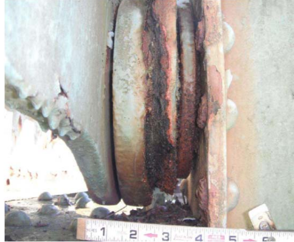
Pack Rust with Section Loss at Lower Chord Pin.
