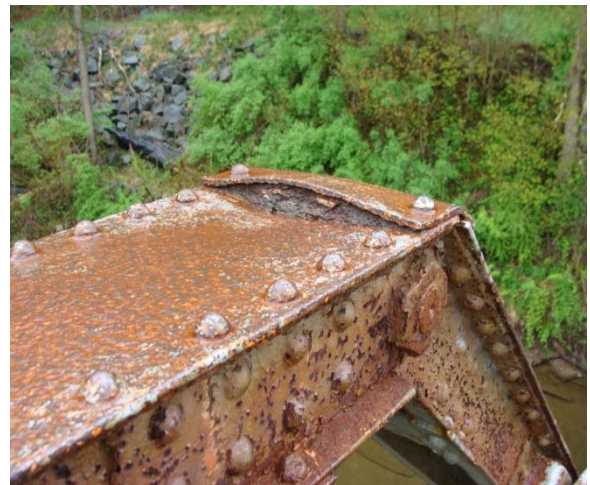
Pack Rust at Top Chord.
