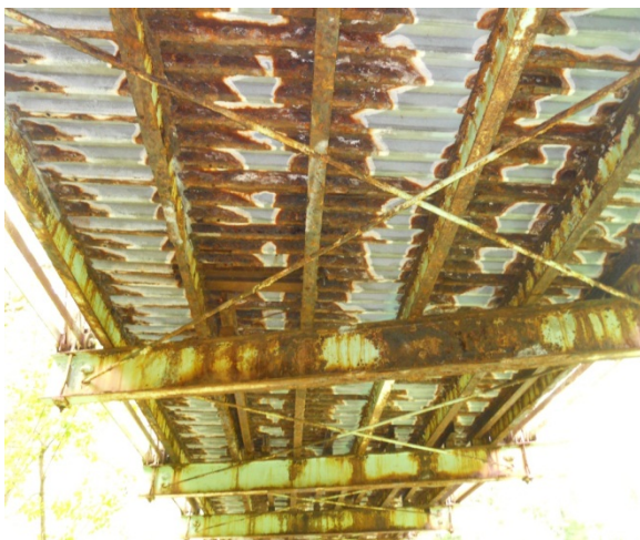
Underside of Bridge Showing Deterioration to Floor System due to Leakage through Bituminous Filled Pan Deck System.
