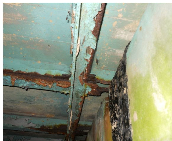
Severe Stringer Deterioration at Abutment due to Leaking Deck Joint.
