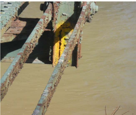
100% Section Loss of Truss Vertical Web at Floorbeam Connection.
