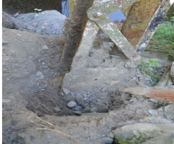
Truss Bearing Covered with Dirt and Debris.
