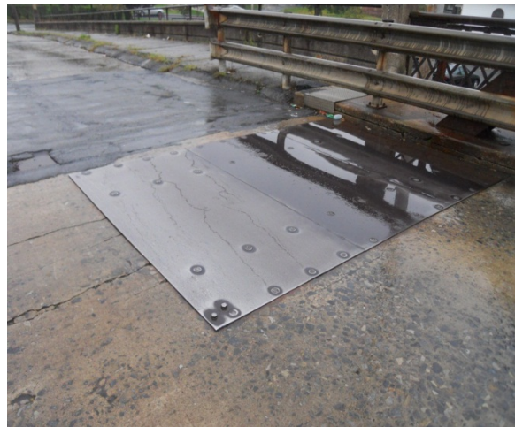
Large Area of Plated Over Concrete Deck Deterioration.
