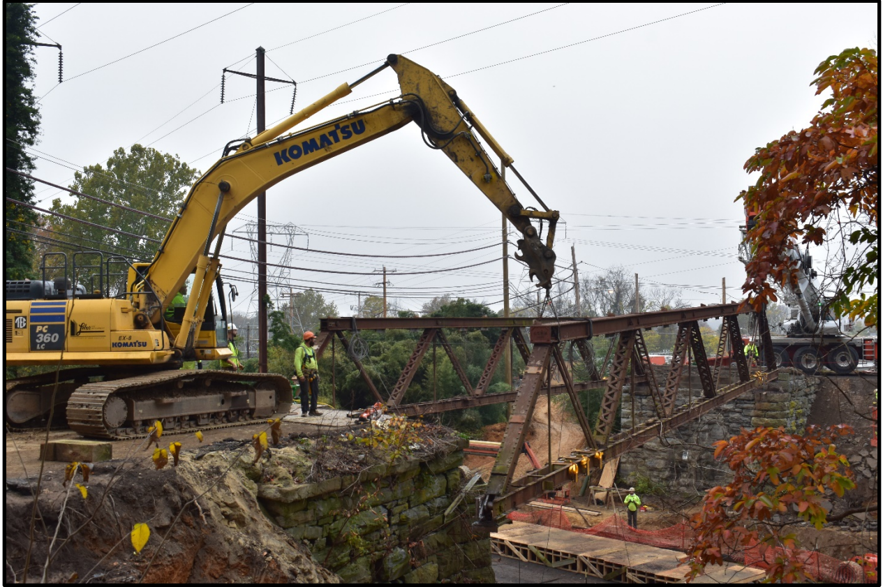
Photo 3: Howellville Truss Bridge in Tredyffrin Township as one truss is lifted off its stone abutments in preparation for the move to Tioga County.
