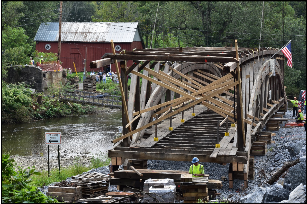
Photo 6: Dreibelbis Station Covered Bridge, removed from its original abutments. One abutment is seen in the left center of the photo, with several of the onlookers to its right.
