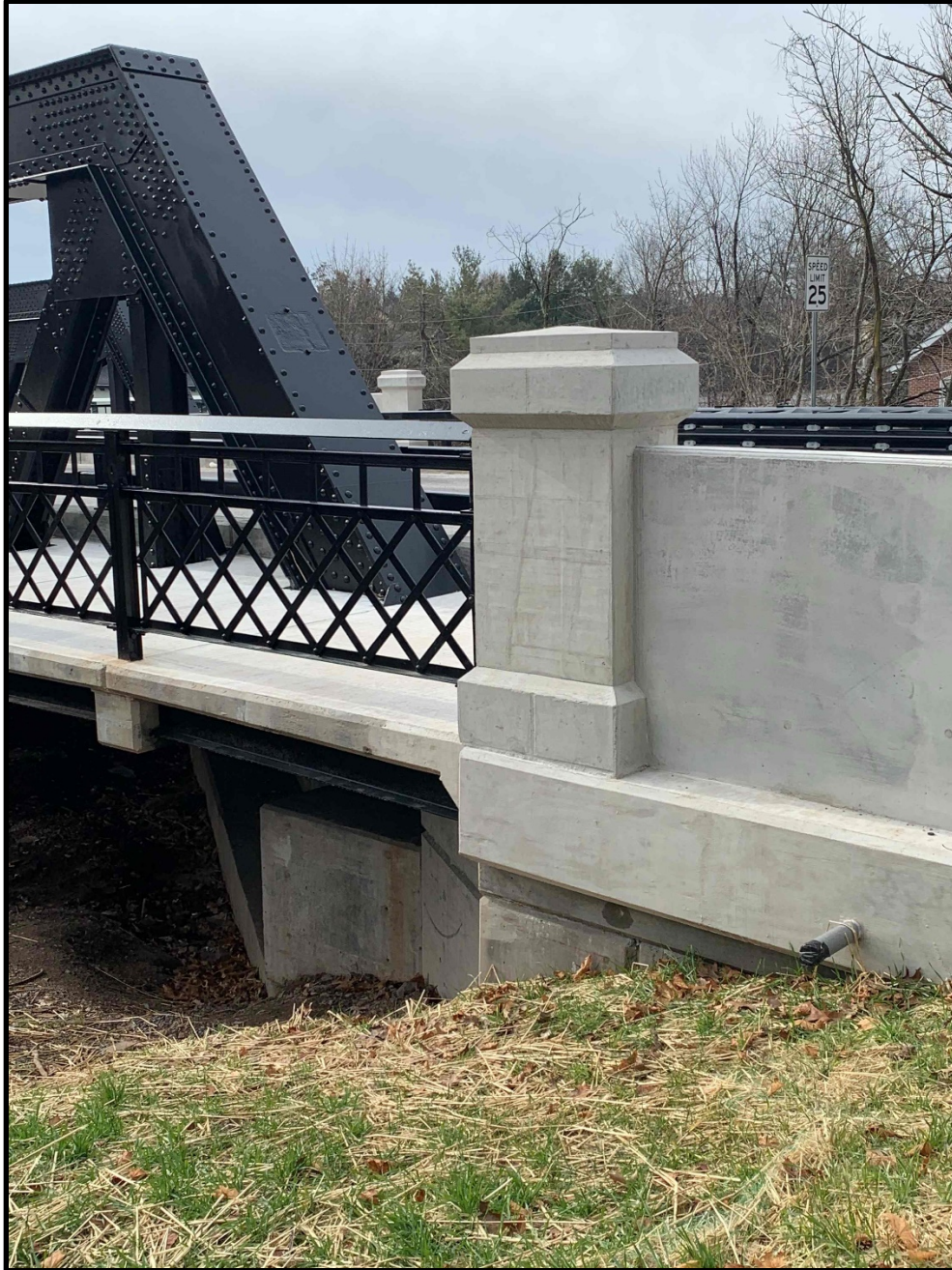
Photo 4: Main Street Bridge over SEPTA in Sellersville Borough, post-rehabilitation. The bridge is individually eligible and contributes to the Sellersville Historic District.
