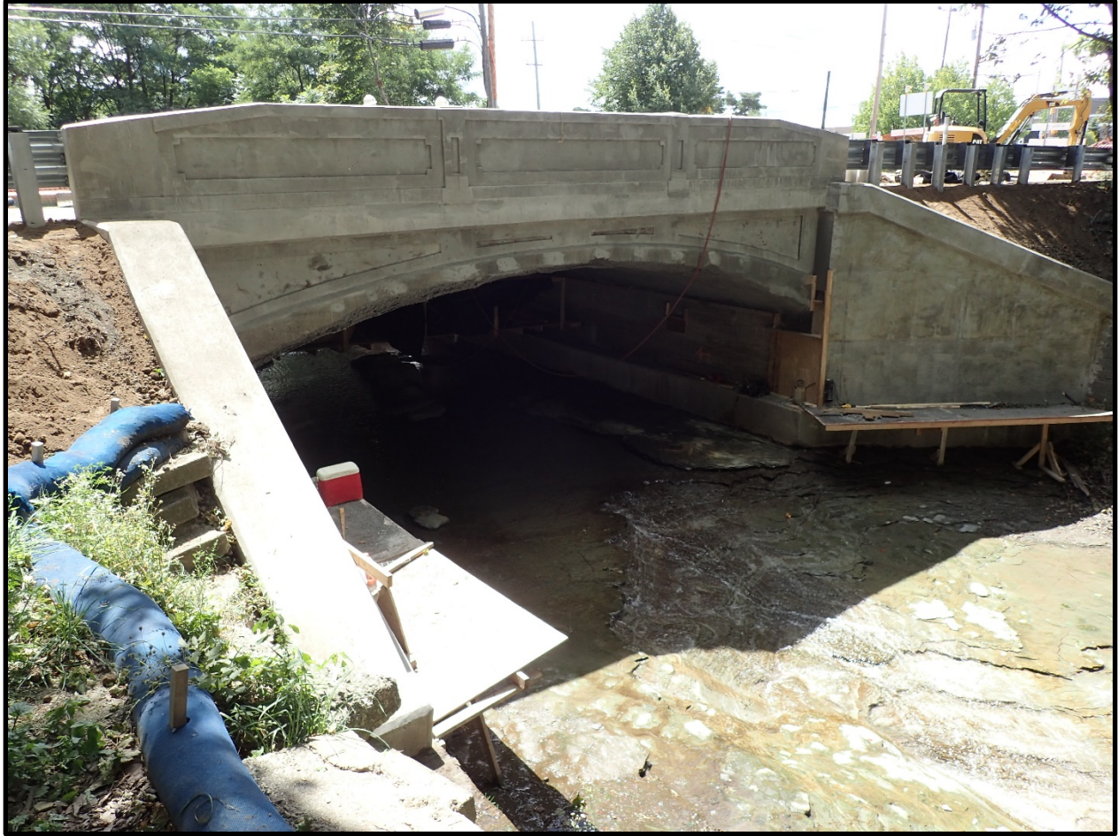
Photo 1: Main Street Bridge over Four Mile Creek, rehabilitated arch with new parapets similar to the historic design.
