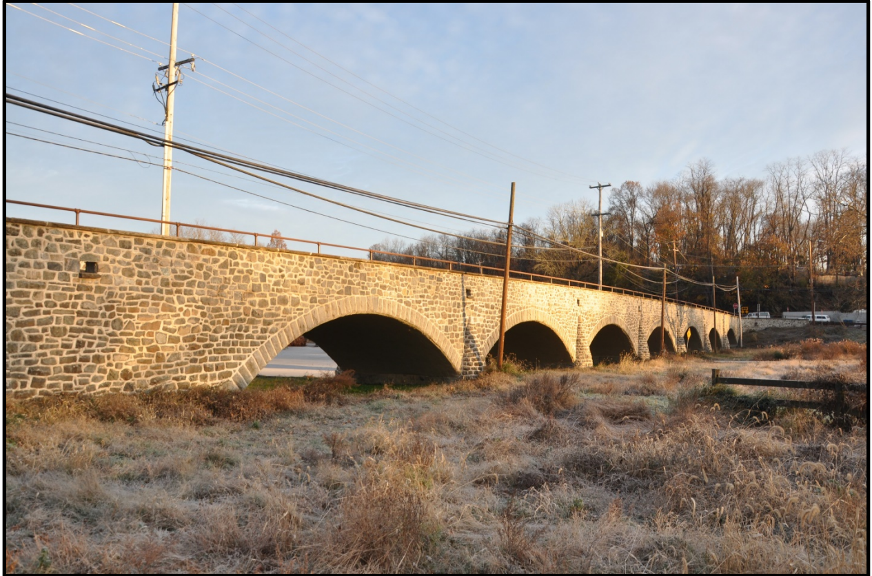
Photo 2: Lenape Road Bridge over Brandywine Floodplain, a National Register-listed bridge after rehabilitation.
