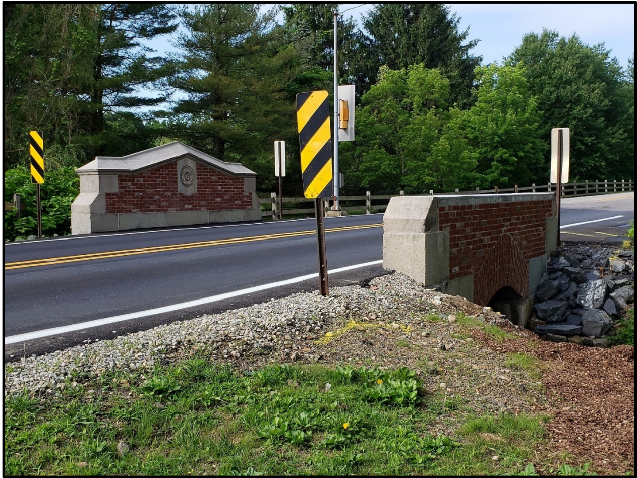
Photo 5: Bryn Mawr Avenue Bridge over Meadowbrook Run in Radnor Township after parapets were reconstructed with a concrete core.
