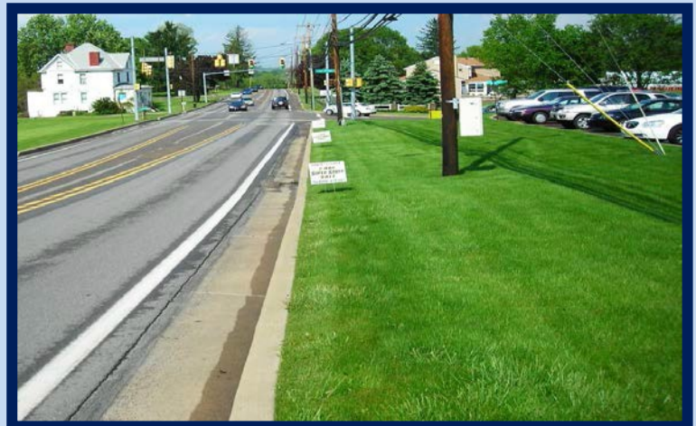
Figure 1.4.2- New enclosed surface storm water installed with curb gutter as part of widening for left turn lane.
