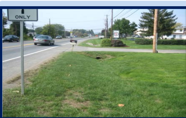
Figure 1.1.1- Pipe conveys water under driveway from storm water feature.
