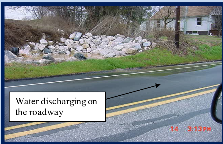
Figure 1.2.3- A photo of storm water that is not adequately retained and overflow water ponds on the roadway surface.
