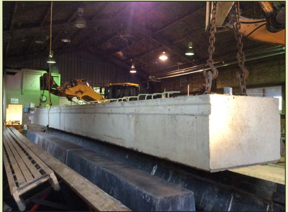
A precast channel beam is lifted from a form at the Crawford County Maintenance facility.
