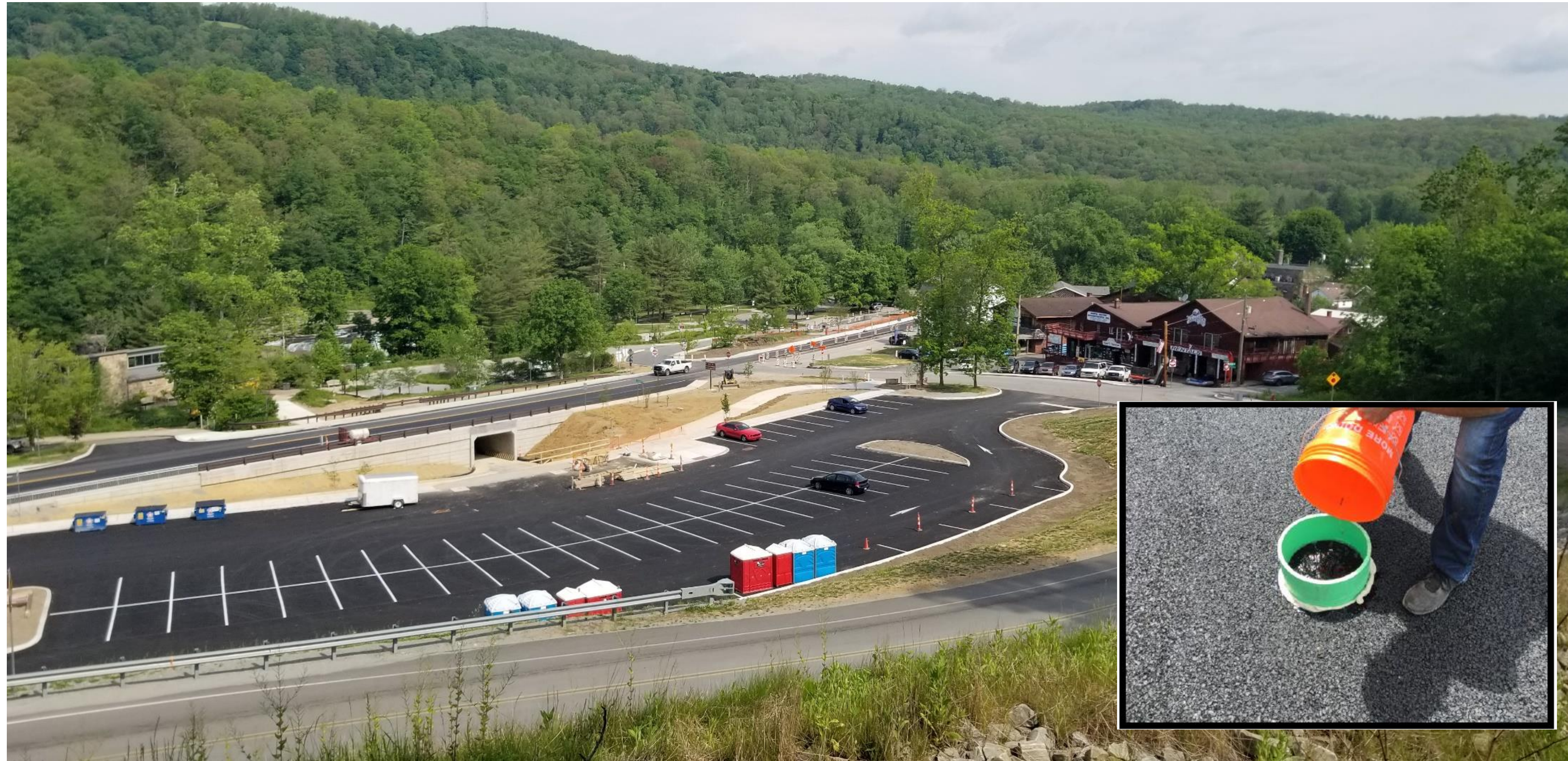
Green Infrastructure Parking Lot
