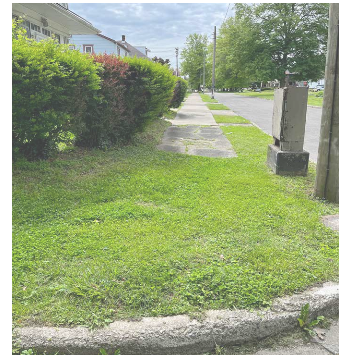
Sidewalk gap on Dunn Boulevard at 2nd Street
